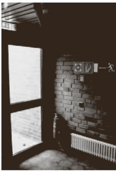
Figure 59: Emergency exist in an administration building, with sign and fire extinguisher (Source: BGI 560)
