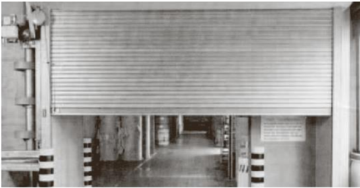
Fig. 60: Rolling shutter gate for fire safety (Source: BGI 560)
